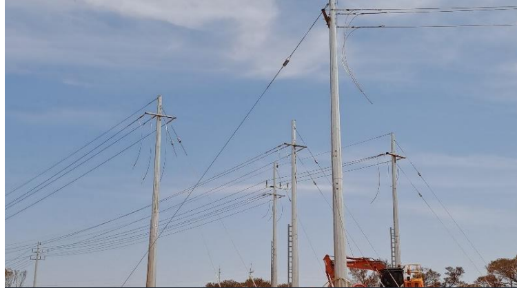
Bellevue Gold 33kV and 11kV Power Line (2023 – Present)
