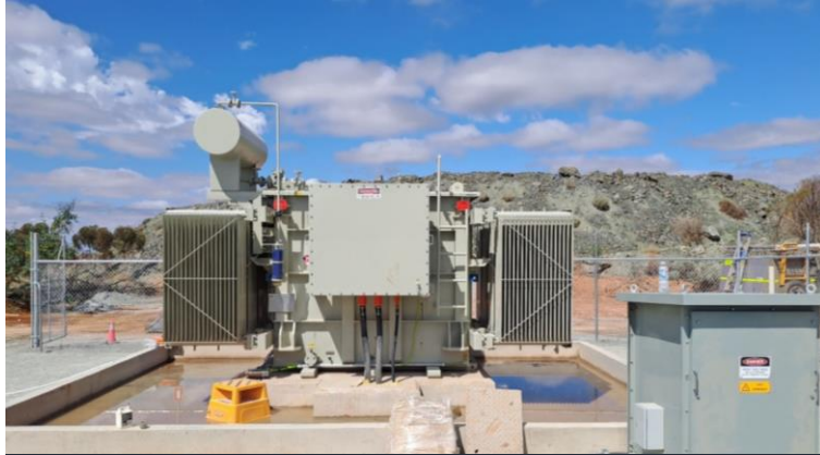
Jubilee 33/11 kV Substation (2023)
